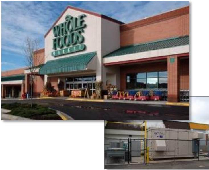
Fuel Cell installed at Whole Foods in Fairfield, CT
